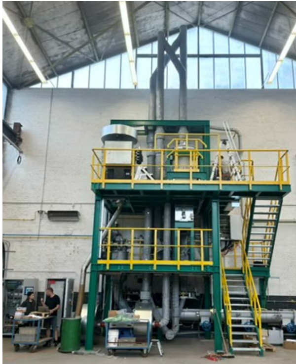
Flash calciner test plant for sample testing & process optimization (operational since 2025)
